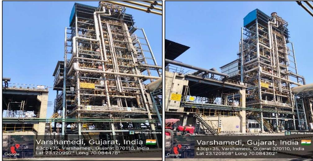
Geo tagged Photographs of Waste Heat Recovery Boiler
