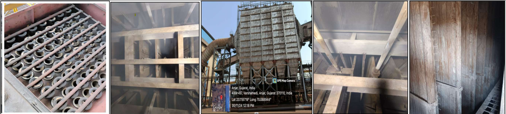
Photographs of the Maintenance of ESP fields & Bags replacement in Air Pollution Control Devices (APCD)
