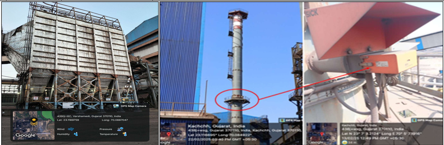
Geo-tagged photographs of Installed APCD's and regular Environmental Monitoring at WML Unit
